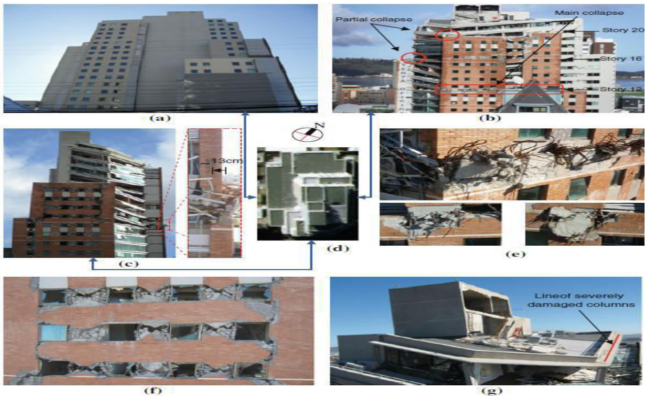
Figure1 Over view of building :(a) West side view ,(b) East side view , (c) South side view and close-up , (d) Plan view , (e) Details of the main collapse at story12 ,(f)Damage in short columns in axis , (g)Overall condition of the 21 st story
